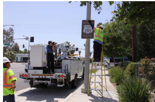
City street crews hang a Historic Route 395 sign on Main Street in downtown Riverside on April 15, 2015.
